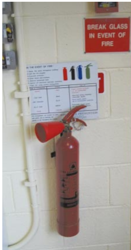
Regulations dictate that fire extinguishers, like all health and safety equipment, must be serviced annually.
